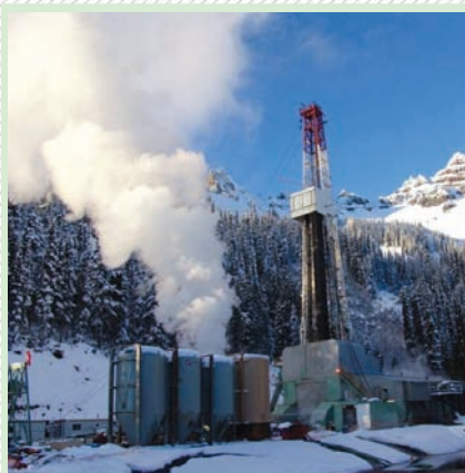
South Meager Geothermal Project near Pemberton, B.C.
