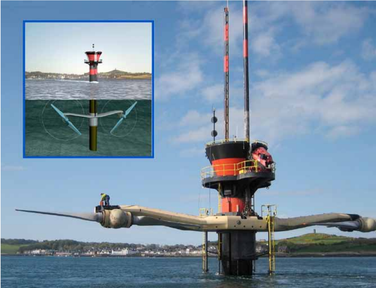
Figure 32 Marine Current Turbine's first generation 'SeaGen' device installed at Strangford Lough, with turbines raised for access
